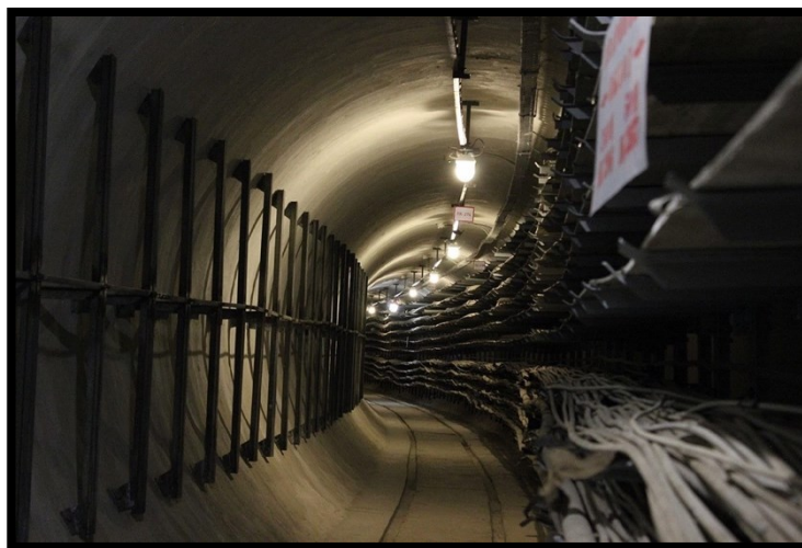
FIGURE 2: IMAGE OF UNDERGROUND COMMUNICATION COLLECTOR. IMAGE RETRIEVED FROM MOSCOW URBAN SERVICES COMPLEX WEBSITE
