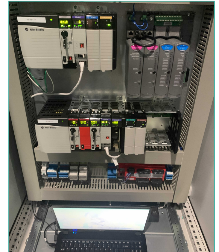
Figure 5: The Dragos Rockwell ICS Range - Panel 2
